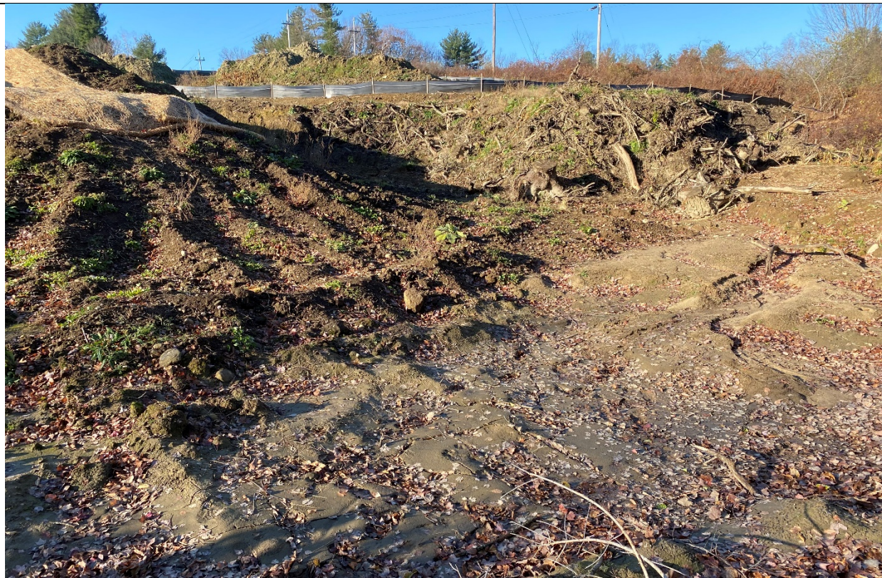
Photo 8: An unstabilized area at the northern site perimeter is eroding, with sediment buildup confined by an ungraded berm. Mr. Vaine stated that this area would be graded and stabilized within 2-weeks.
