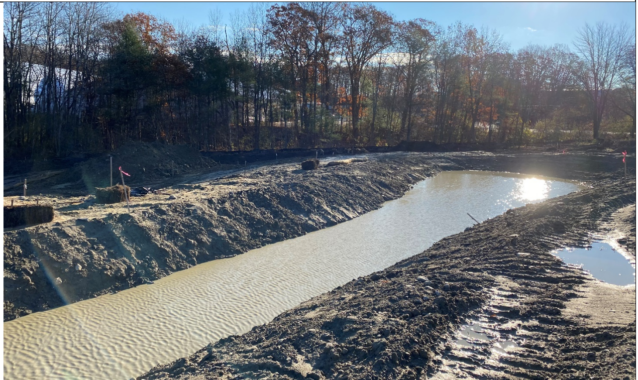
Photo 4: The rough-graded temporary stormwater basin was holding water from recent rainfall. The basin appeared to performing as expected, with no indication that its perimeter berms had been compromised or overtopped.
