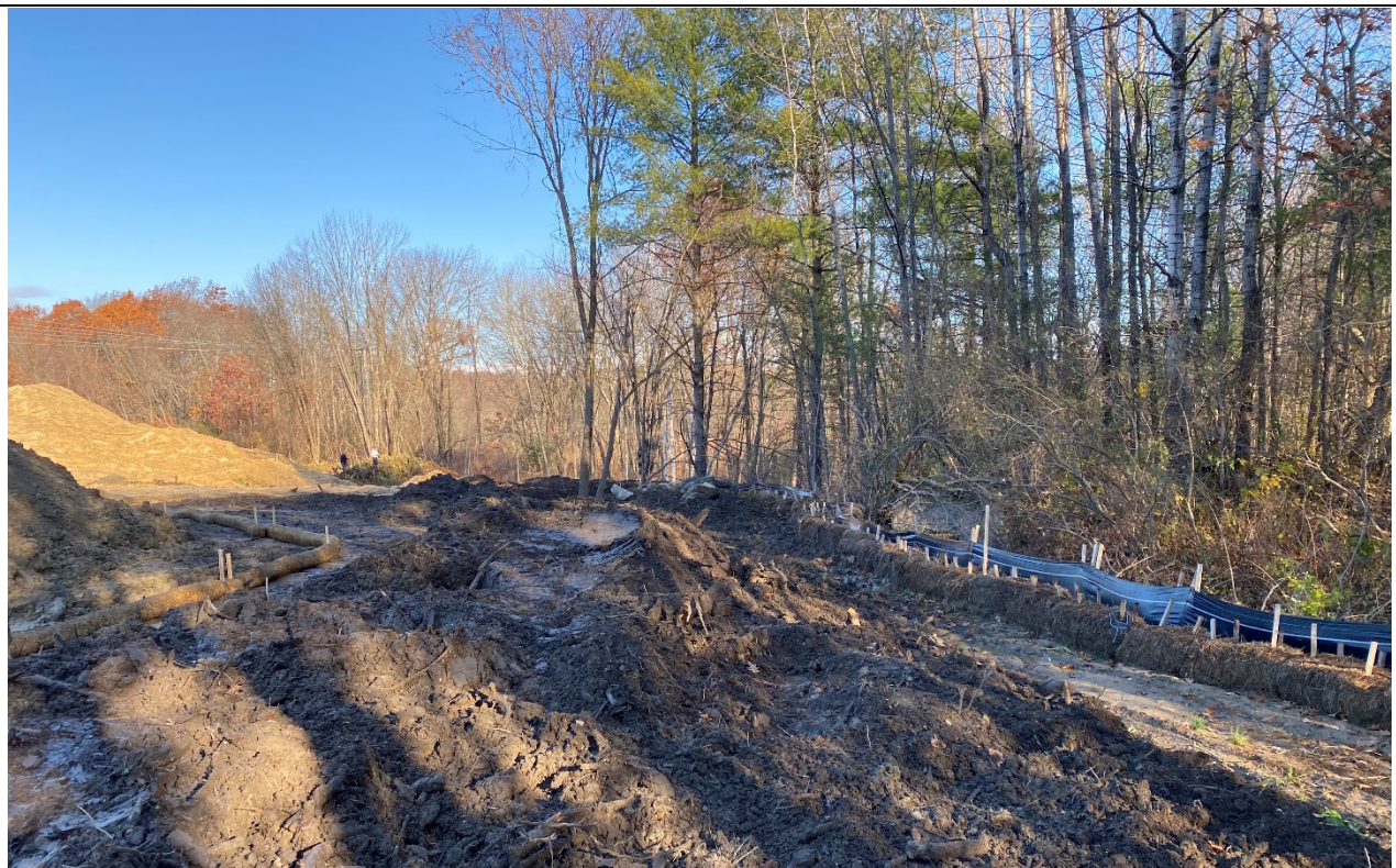
Photo 6: To the east of the stormwater basin, there has been significant progress in removing the berm of earthen material and stumps so that water from the basin can flow to its intended outlet.
