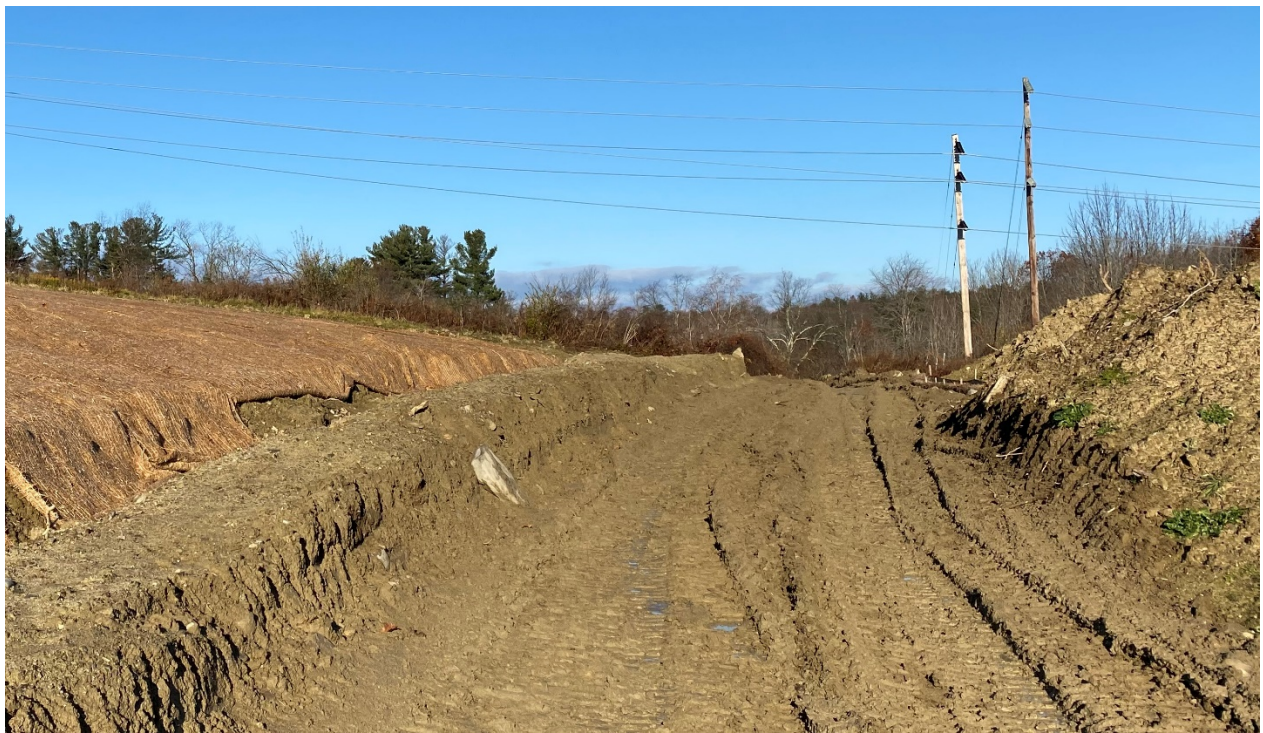
Photo 2: A temporary haul road is in place between the area stabilized with ECB and the area of ongoing work in the vicinity of the stormwater basin.
