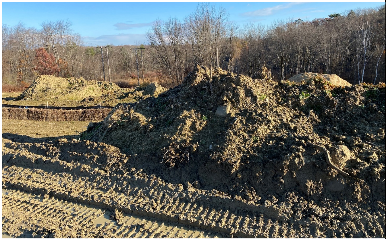
Photo 3: Several loam stockpiles remain unstabilized. Mr. Vaine stated that this loam will be actively used over the next week for ongoing final construction/grading of the sediment basin area.
