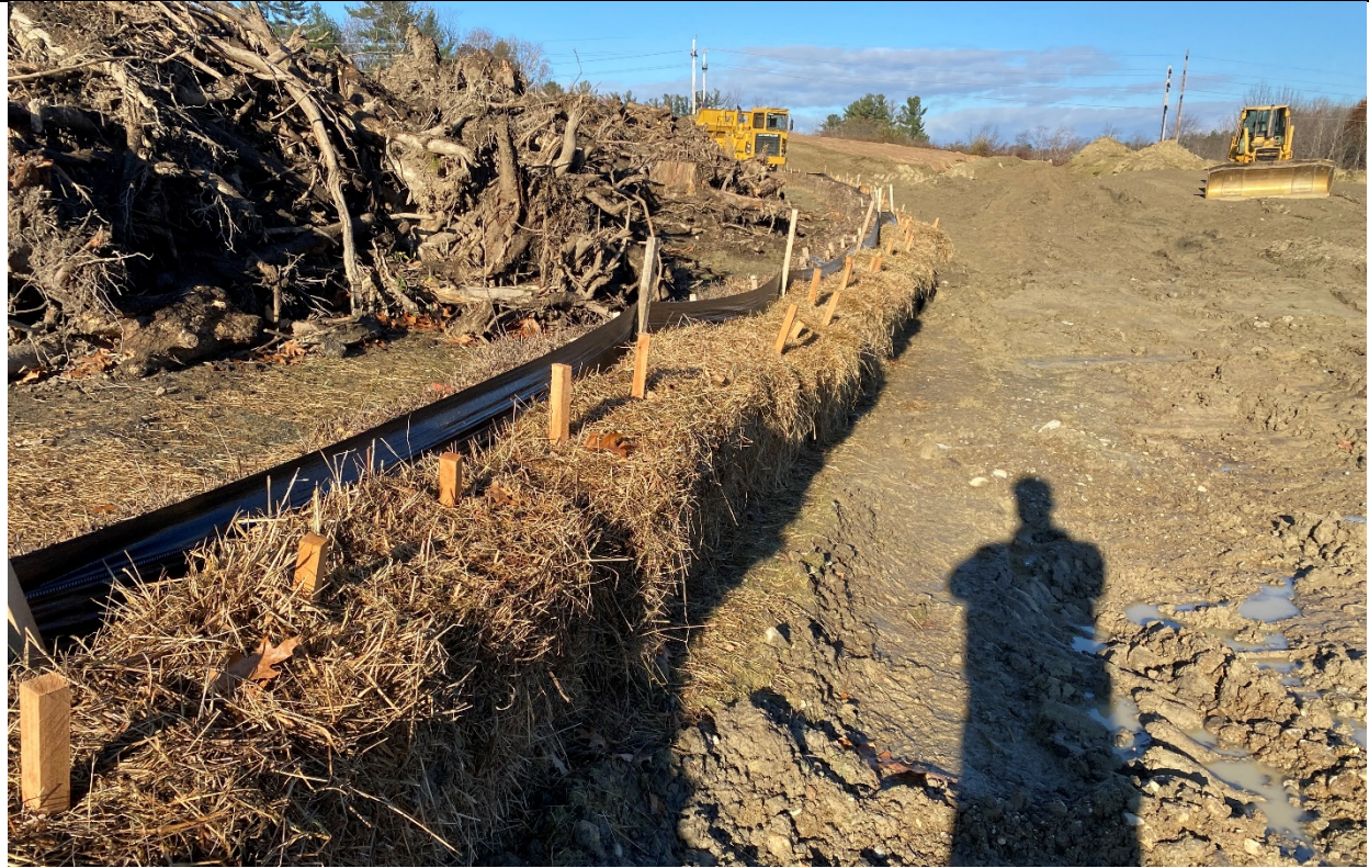
Photo 5: A row of straw bales has been properly installed on the downslope side of the silt fence within the interior of the site. Silt fence/straw bales along the downgradient (eastern) limit of disturbance were in good condition
