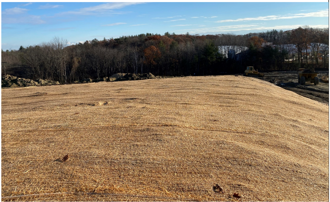
Photo 1: ECB has now been installed over most of the area to the west of the stormwater basin.
