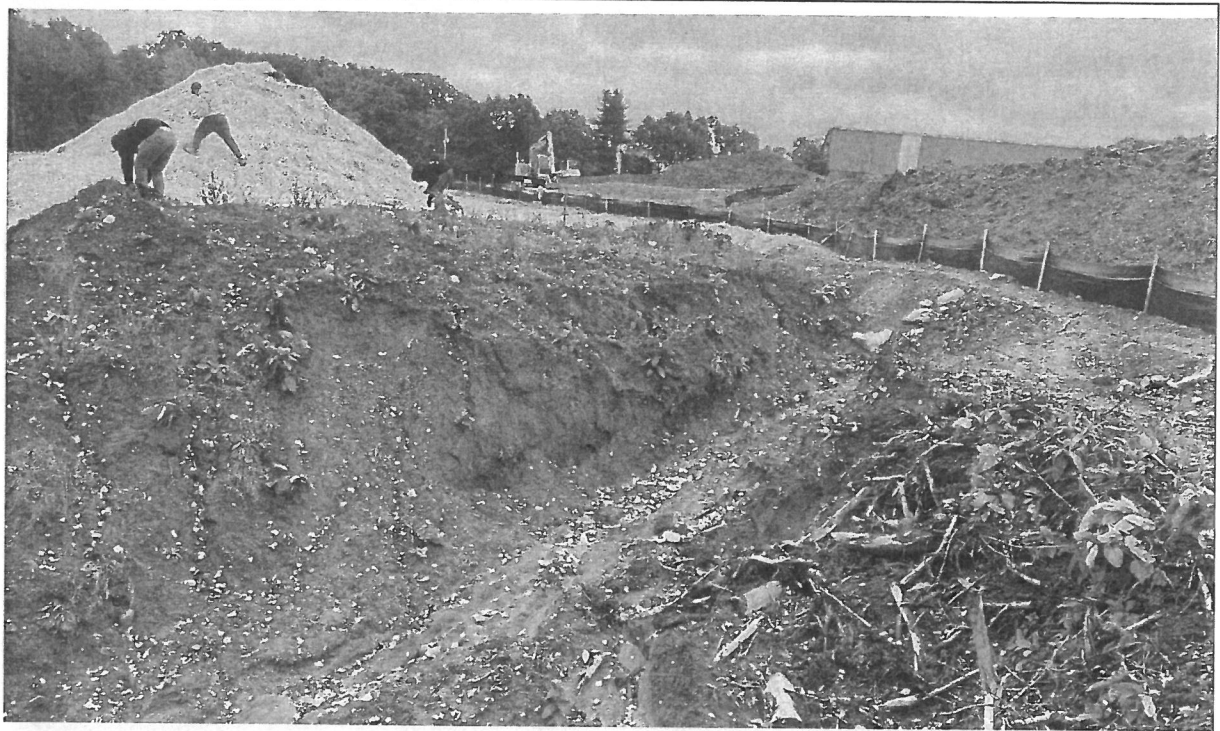
Photo 3: Erosion control blanket being installed in the wetland buffer zone area without prior surface preparation or hydroseeded. Areas upgradient of the silt fence (upgradient of the buffer zone) have only been hydroseeded.
