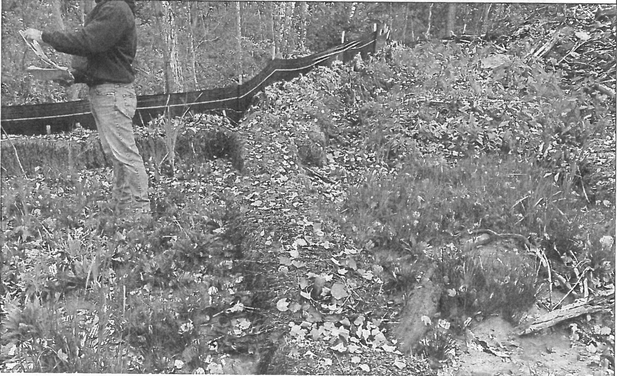
Photo 4: Silt fence/straw bale controls have been installed incorrectly, with strawbales on the upgradient side of the fence instead of the downgradient side as specified in the plans. Straw bales along the fence line in the photo (adjacent to wetland boundary) are in poor condition and should be replaced.
