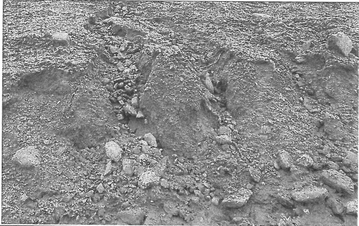
Photo 1: Hydroseed/mulch was applied, but had patchy ground coverage and was applied without surface preparation. The mulch is not expected to provide adequate stabilization for disturbed areas where no other measures are currently proposed. It is likely too late in the season to expect much of the seed to germinate.
