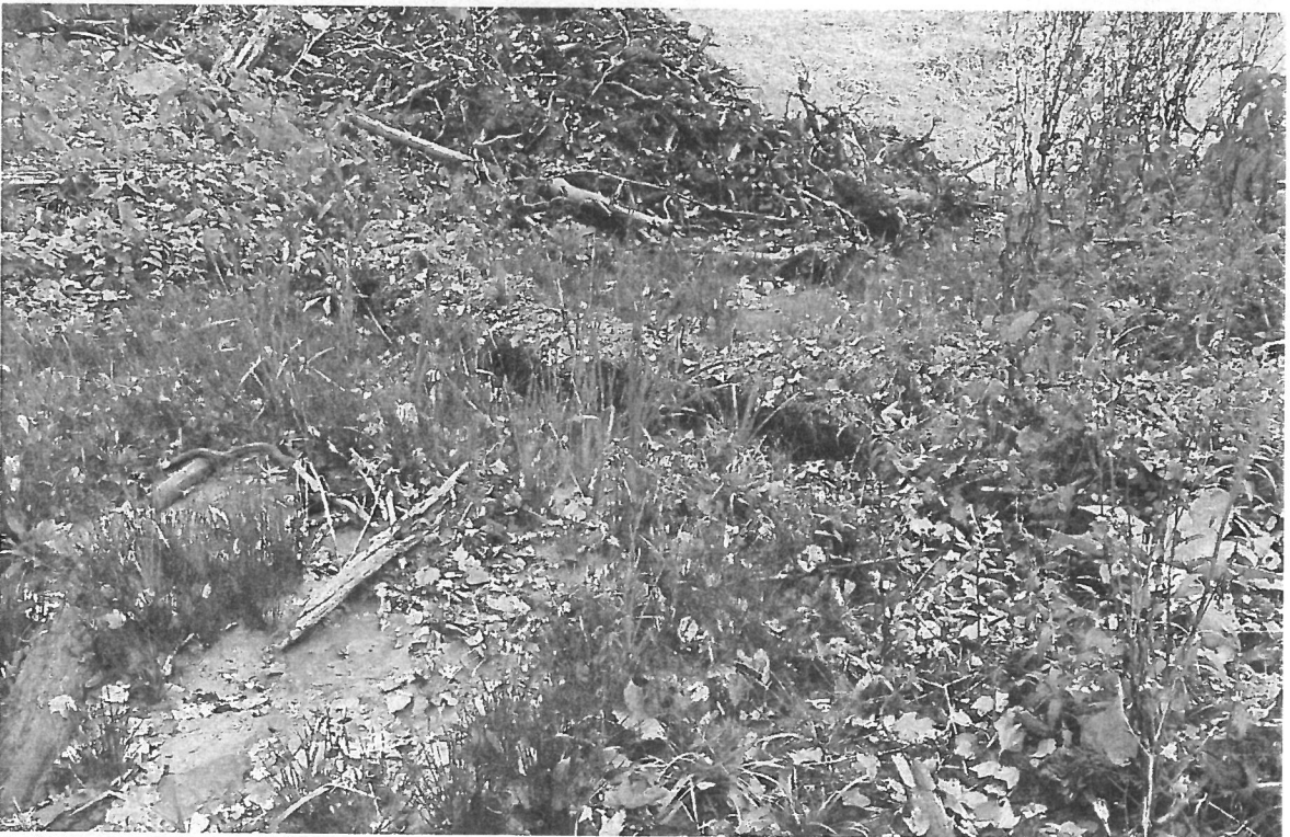
Photo 6: View from wetland area near flag W20, towards point of discharge resulting from presence of berm. This area is currently protected only by several staked straw bales.
