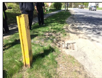
Image 5: Sand buildup around existing catch basin along the southerly side of Main Street
