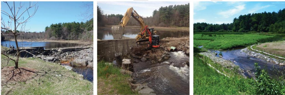
Left to Right: Dam before removal; dam at the start of removal; and Wekepeke Brook after removal.
